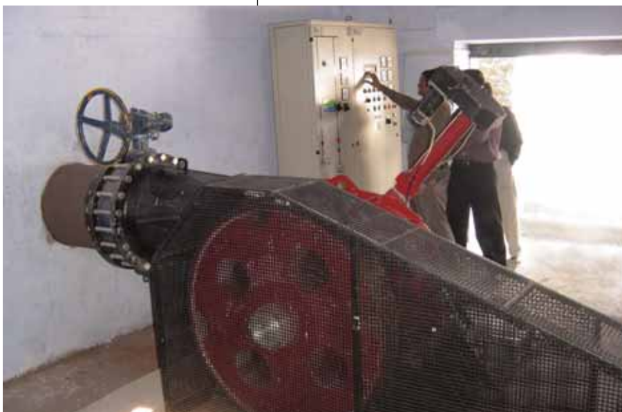
A micro-hydropower turbine at the Kanva Ashram scheme, Uttaranchal, India.
